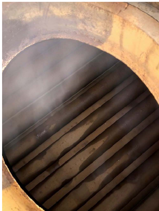
Figure 8. Boiler tubes during inspection at Bear Republic Brewing in 2022, showing unscaled tubes in good condition.
